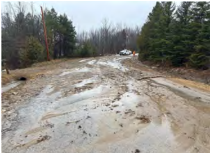
Harbour Beach Road Flooding, March 2026
