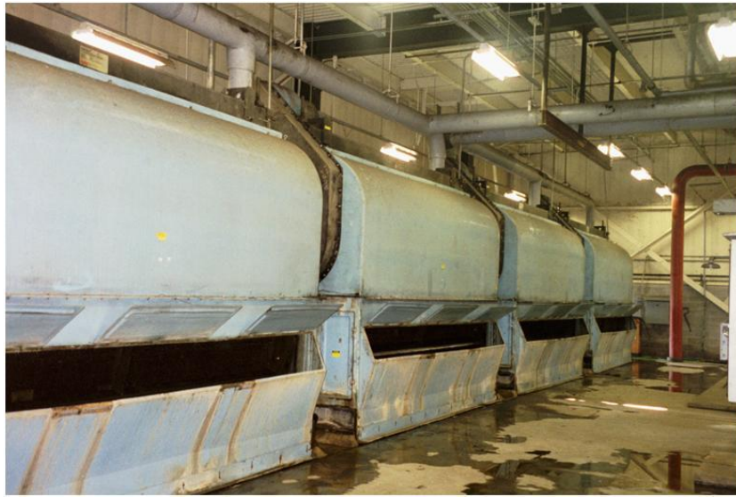
Figure 4-15 Typical Through-flow Traveling Water Screen Arrangement
